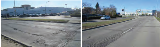
Roads in need of renewal
