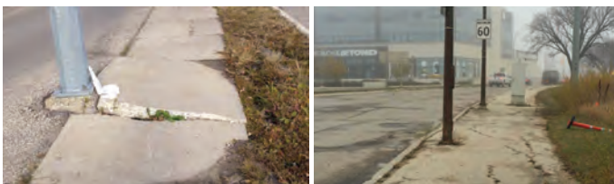
Sidewalks in need of repairs
