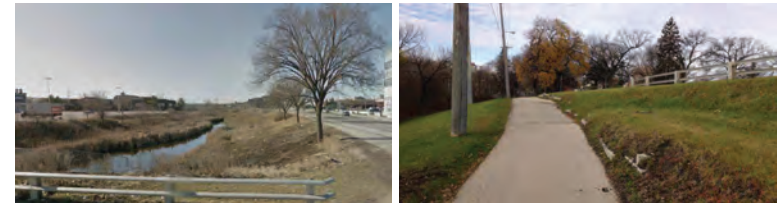
Omand's Creek bank in need of stabilization
