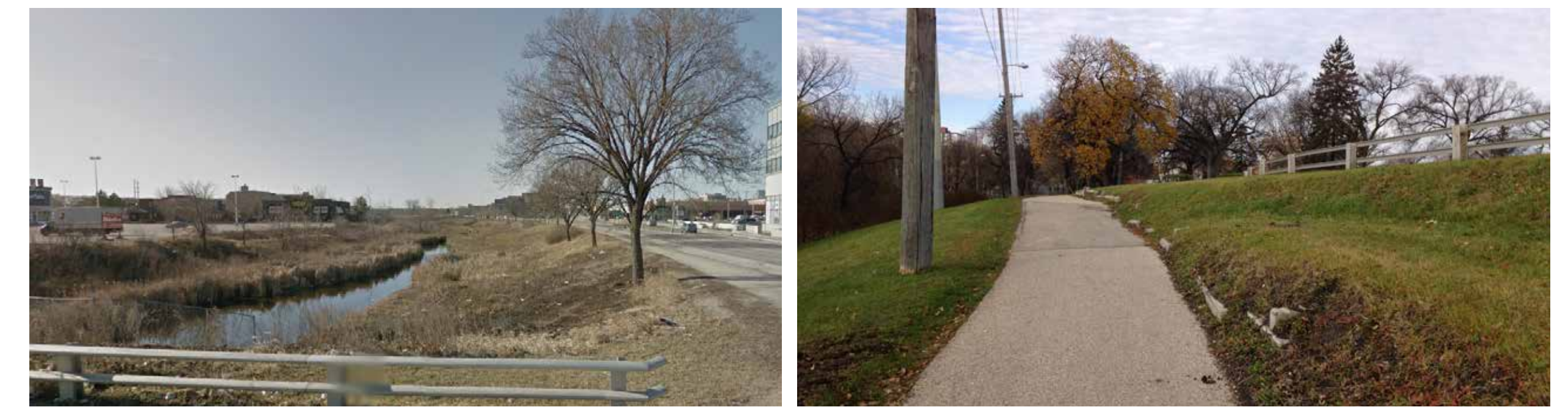
Omand's Creek bank in need of stabilization
