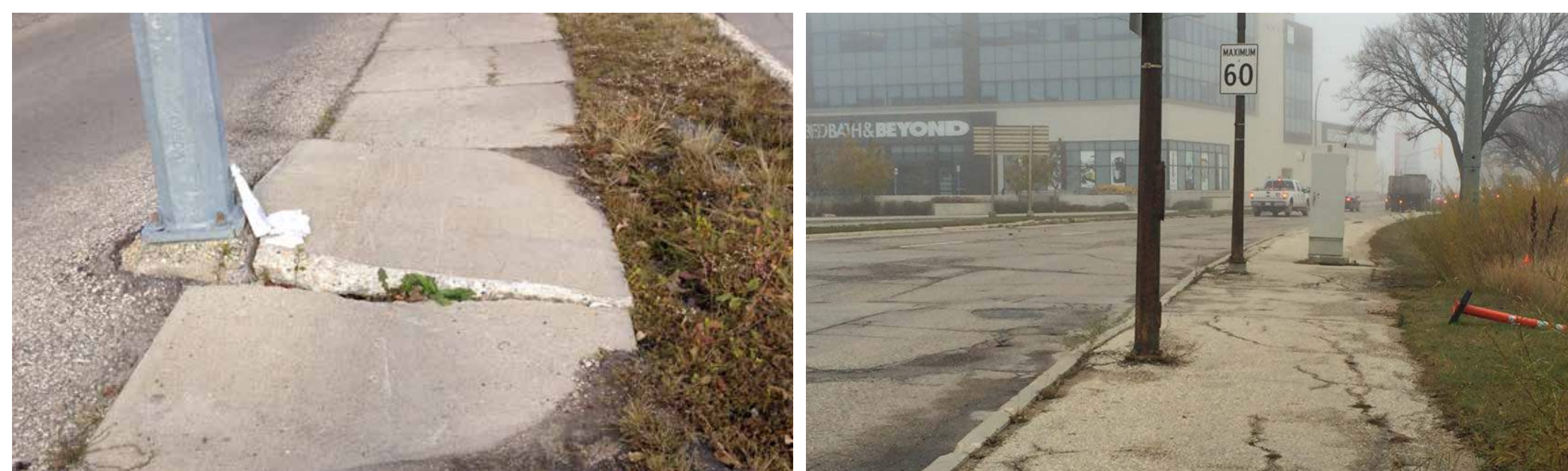
Sidewalks in need of repairs
