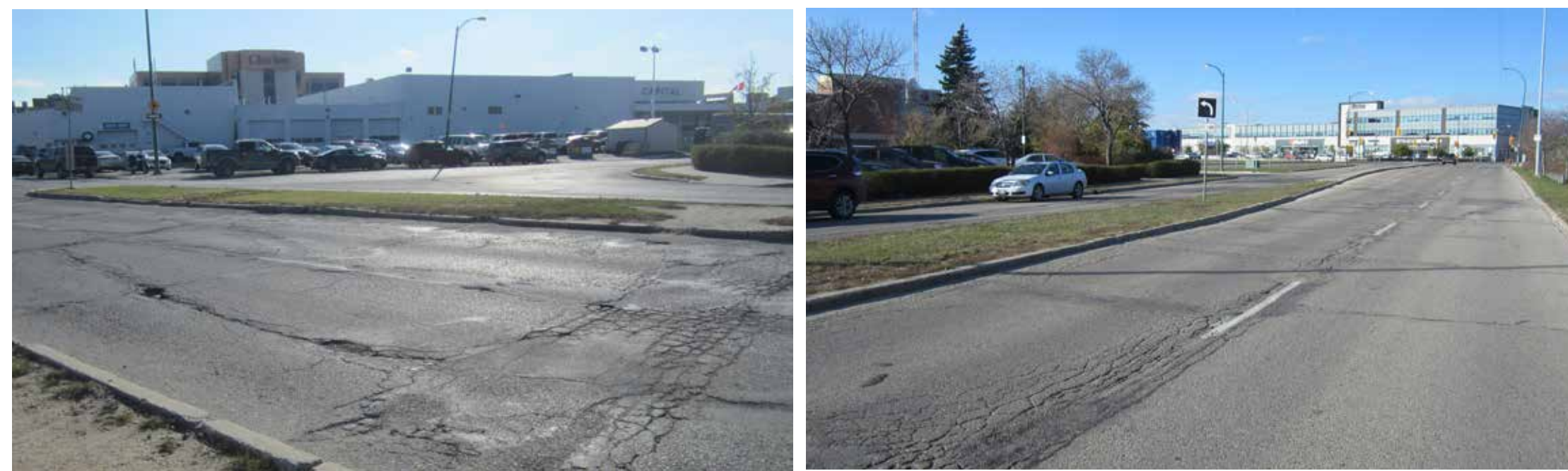
Roads in need of renewal
