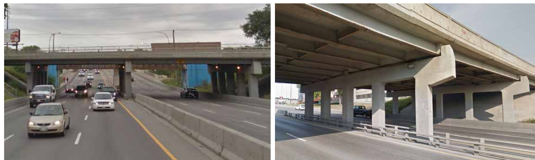
Existing overpass and piers in need of repairs
